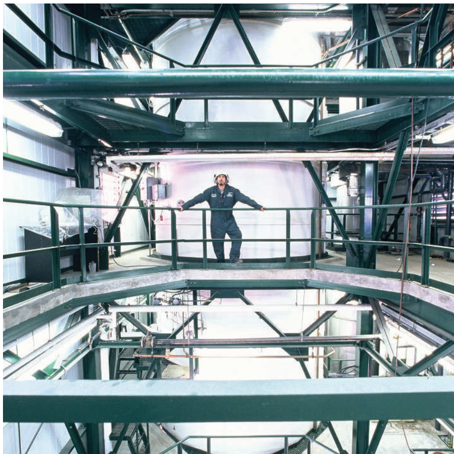
Plant processing: logen's enzyme fermentor, a later stage of turning cellulosic feedstock into ethanol.
